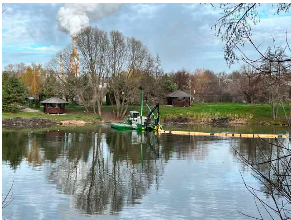
Figure 13. Extraction of bottom sediments by the Watermaster dredger in the Vezelka River in Belgorod (2 km upstream of the gauging station) as part of the implementation of the Program for Clearing and Rehabilitation of the Rivers of Belgorod Oblast (November 2022).
